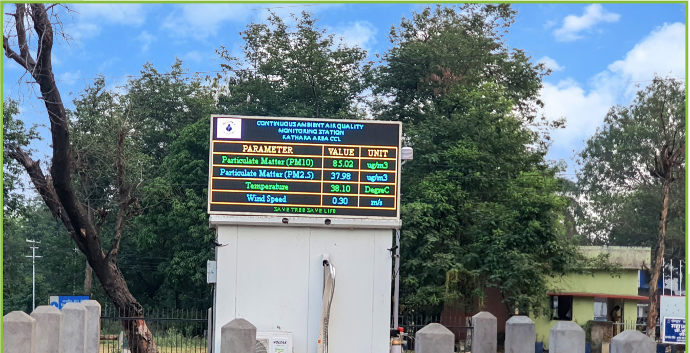
View of CAAQMS system at Kathara Area
