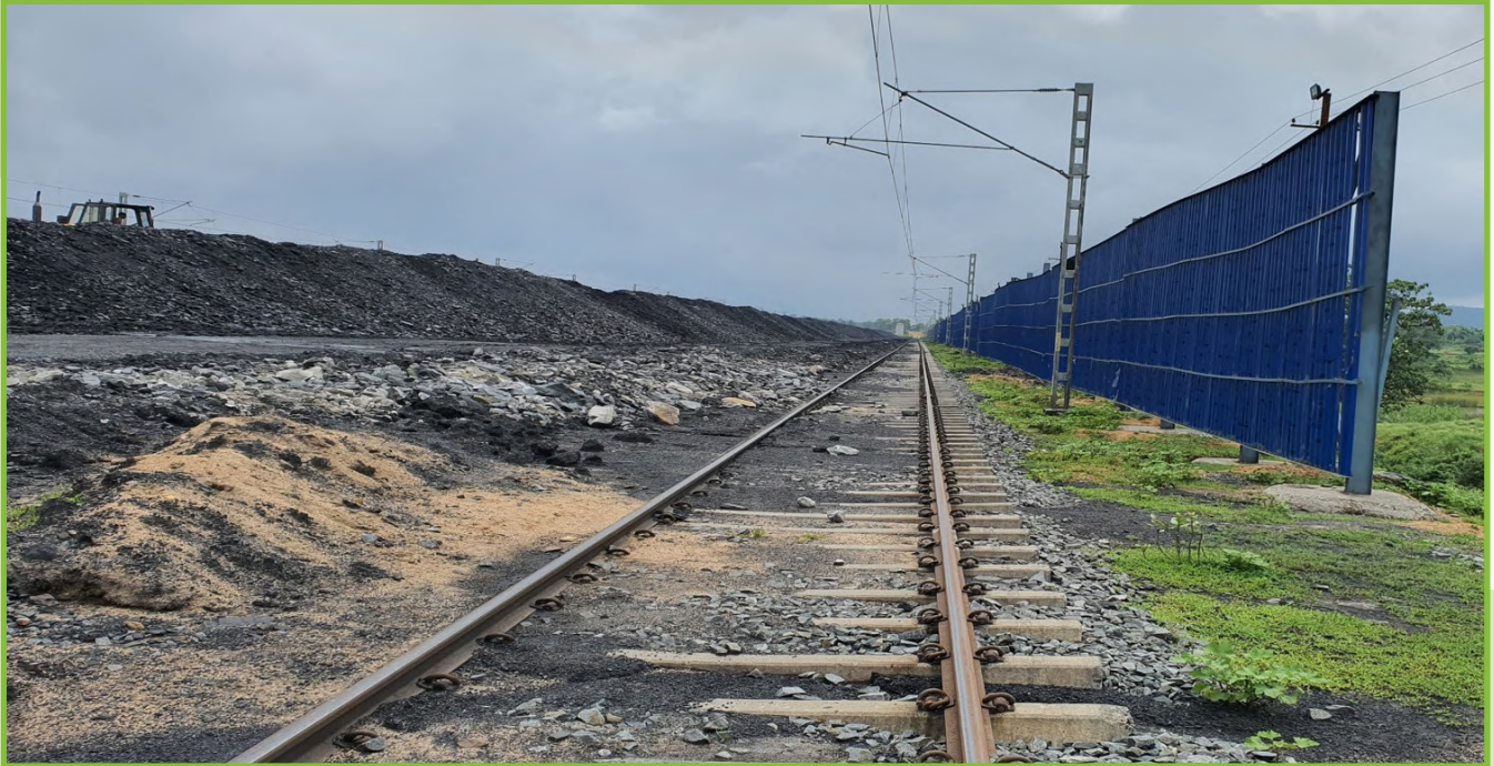
View of Wind Breaking System installed at Piparwar Railway Siding
